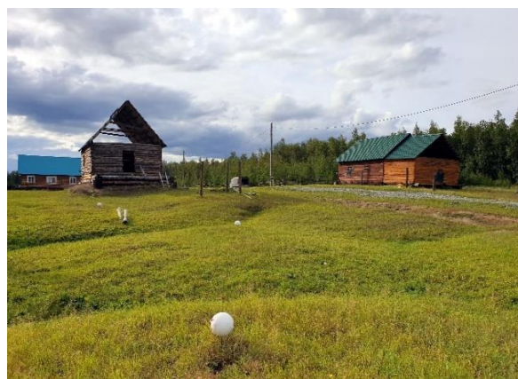
Fig. 24. Building freeze in areas where thermokarst processes have actively developed in recent years, Third arable land micro-district, Ulakhan-An village, August 2022. Photo by A.A. Suleymanov.
