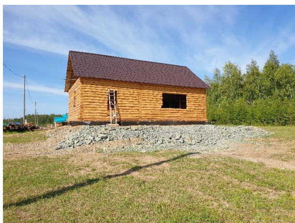
Fig. 40. Adaptation of construction technology to the conditions of permafrost degradation: building a house on a bedrock fill and a metal frame as a foundation, Ulakhan-An, August 2022. Photo by A.A. Suleymanov.
