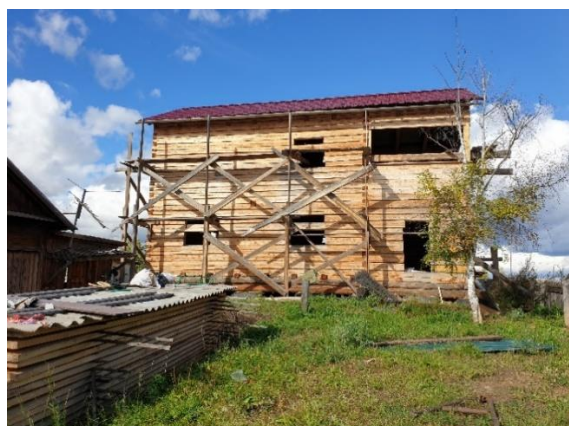
Fig. 38. Adaptation of construction technology to the conditions of permafrost degradation: building a house on old car tires in compliance with the principle of a ventilated underground, Yunkyr, September 2022. Photo by A.A. Suleymanov.
