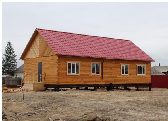
Fig. 39. Adaptation of construction technology to the conditions of permafrost degradation: building a house on a pile foundation, Amga, September 2022. Photo by S.A. Grigoryev.
