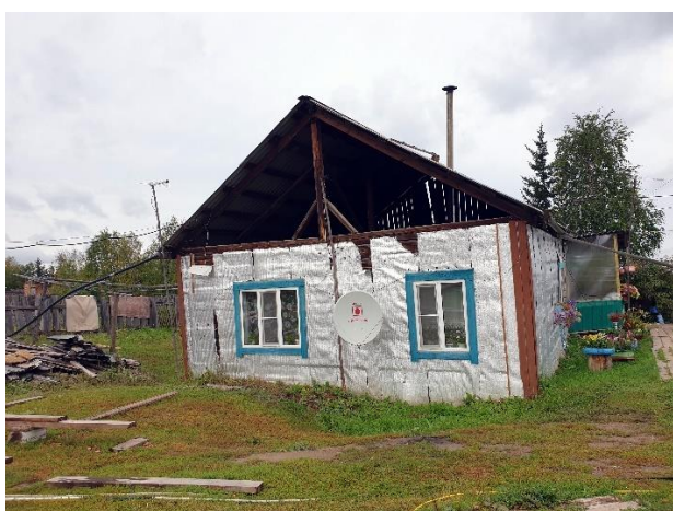
Fig. 25. Consequences of permafrost degradation: the owner of this house had to take a loan for building on a new site and reconsider plans for retirement, Yunkyur, September 2021. Photo by A.A. Suleymanov.
