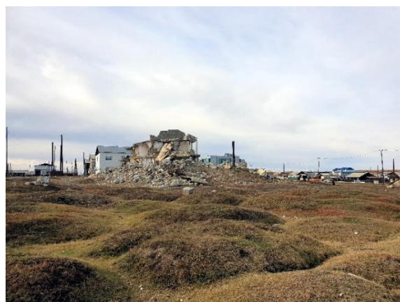
Fig. 45. Remains of the “Experimental house” built without a pile foundation, Amga, September 2021 Photo by A.A. Suleymanov.
