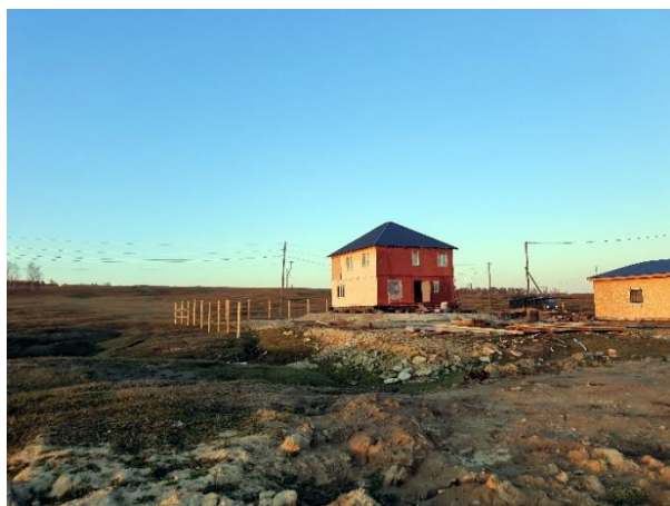
Fig. 36. Construction of houses in areas with active thermokarst processes. According to the owner of the plot, the backfilling in the photo cost more than 300 thousand rubles, Chapchylgan village. September 2022. Photo by A.A. Suleymanov.
