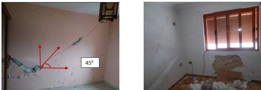
Fig. 24 Diagonal cracks extending over the height of the wall (left), spandrel damage patterns below the openings
