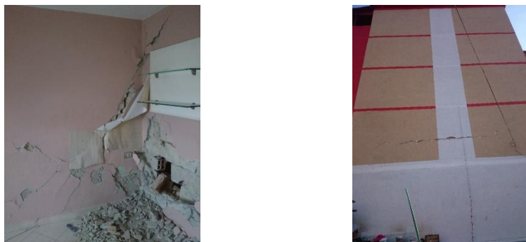
Fig. 25 Heavy cracks (more than 3 cm separation) on load bearing walls and extensive damage on non- load bearing wall (left), serious damage observed on outer facade of the building in lower stories (right)
