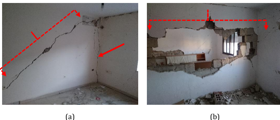
Fig. 11 (a) Extensive shear crack on load bearing wall and separation of two orthogonal masonry walls, (b) Heavily damaged partition wall in an URM building
