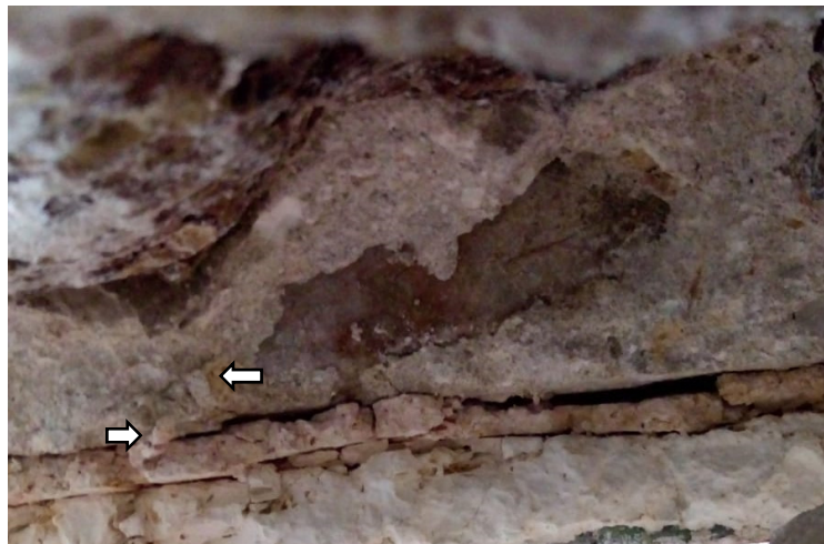
Fig. 3. The figure represents an example of parallel detachment between the brickwork and the arriccio (←) and between the arriccio and the mortar bed(→).The image was taken from the base of the mosaics, after the removal of the marble cornice.
