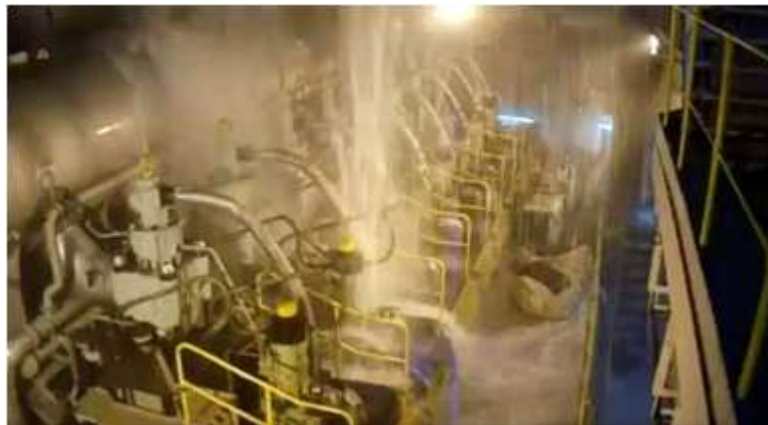
Figure 3: Ship Scrubber System Failure Causes Flooding of Engine Room.
