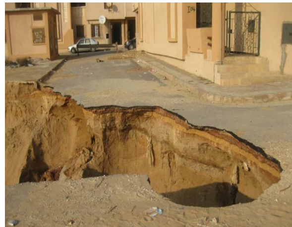
Fig. 4 – Collapse of natural embankments
