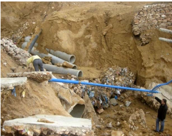
Fig. 3 – Destruction of the retaining walls
