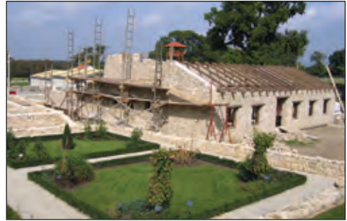
Figure 18. Work in progress reconstructing a Roman private stone house using original materials (2005). (Franz Humer, Haslau a. d. Donau).
