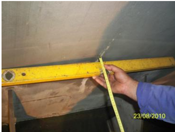
Figure 2. Movement of the bed sheets by 30mm over a length of 1m
