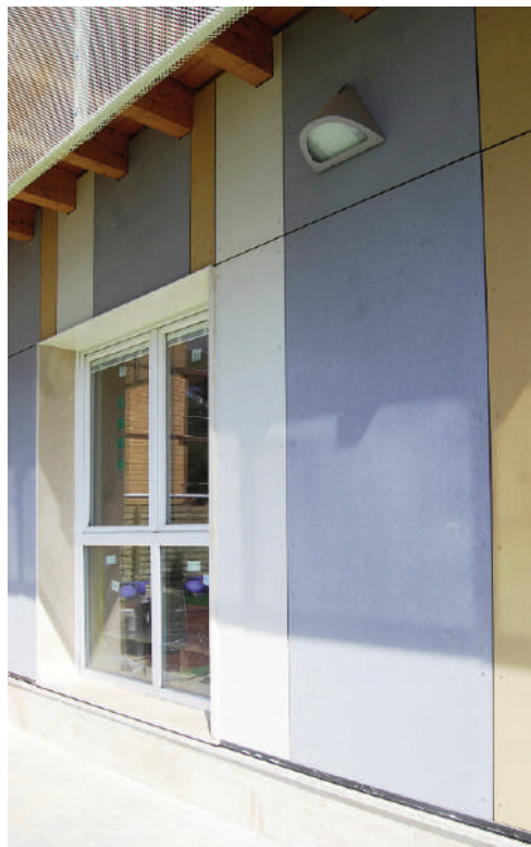
Fig. 12, 13 - Details: The substructure of the ventilated façade in fiber-cement slabs, made with wood slats; The façade covered in dry-mounted fiber-cement slabs, with the effect of solar shading given by the metal mesh panels (credits: P. Altamura, 2017).
