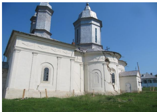
Figure 1 - Failure of church structure by land scouring under the foundation.
