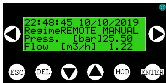
Figure 5. HMI screen and manoeuvring buttons.
