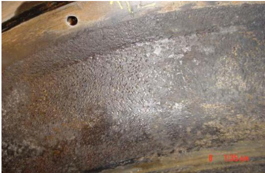
Figure 2. Surface Corrosion Points
