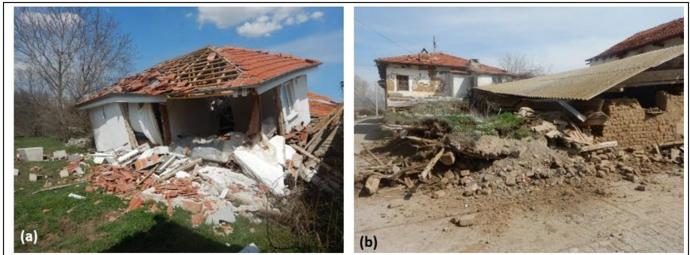
Figure 8(a): Heavily damaged hollow brick structure, (b): Collapsed adobe structure in Kirka village.
