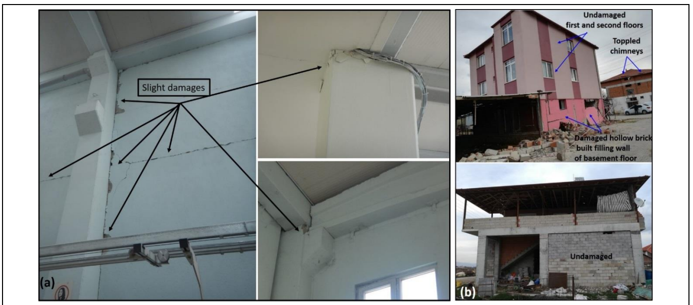
Figure 11(a): Damages on precast concrete modern textile factory structure in Yassihüyük village, (b): Partly damaged three-storey reinforced structure and undamaged single-storey reinforced structure in Apa village.
