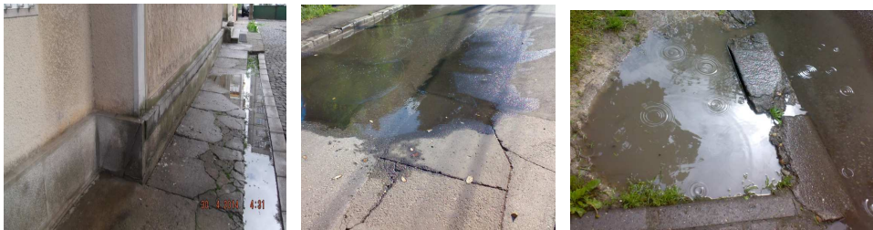
a) building degradation b) roads degradation c) sidewalks degradation
