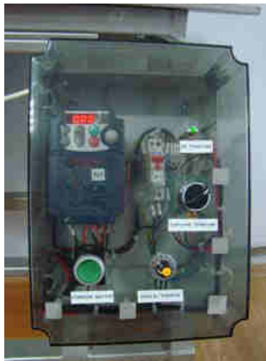
Figure 5. The control panel of the shaking table
