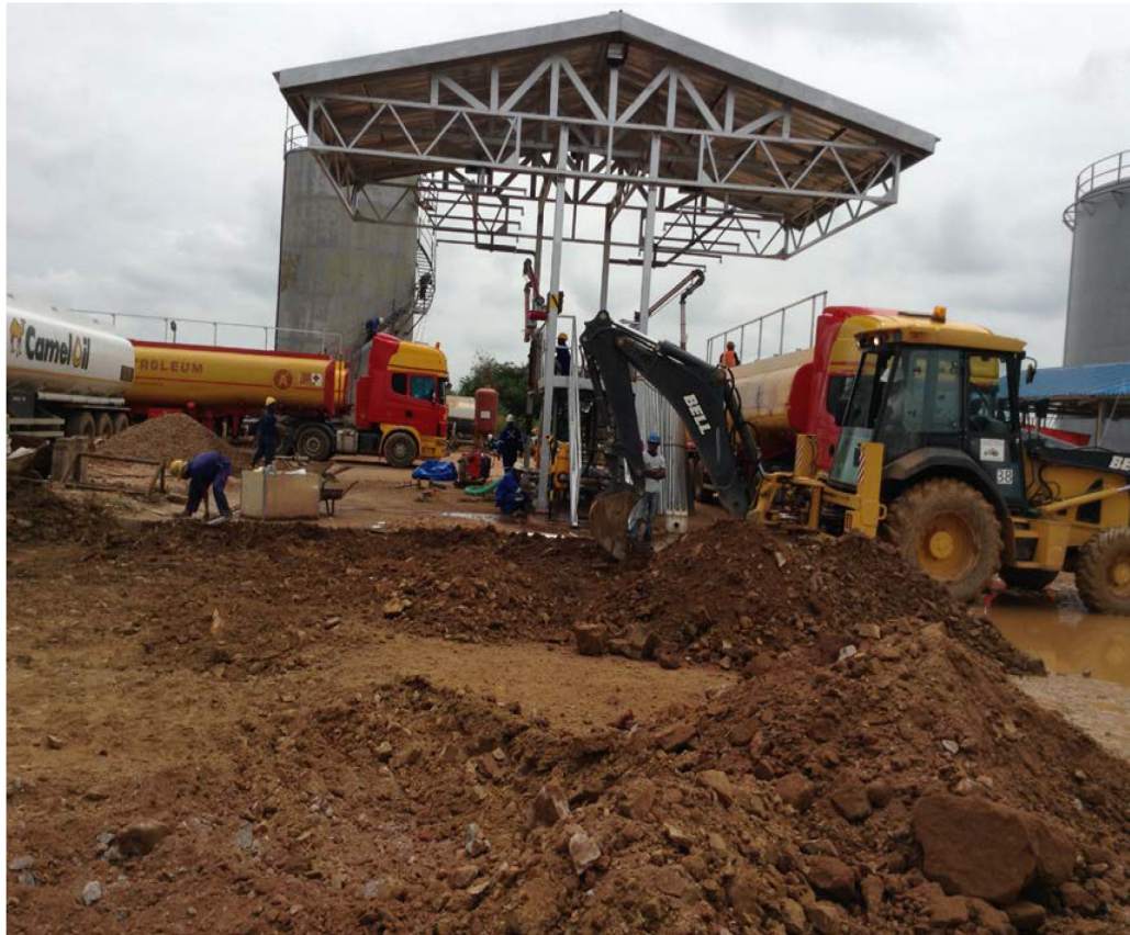
Photo No. 1. Datelines set to finish project where safety is a concern as fuel is offloaded & loaded. Complete construction of tanks and pipelines to alleviate fuel storage issues. Source: 1 st Author.
