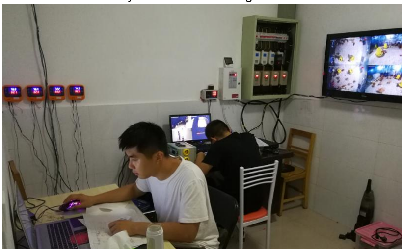
Fig. 2 - Control room and control system
