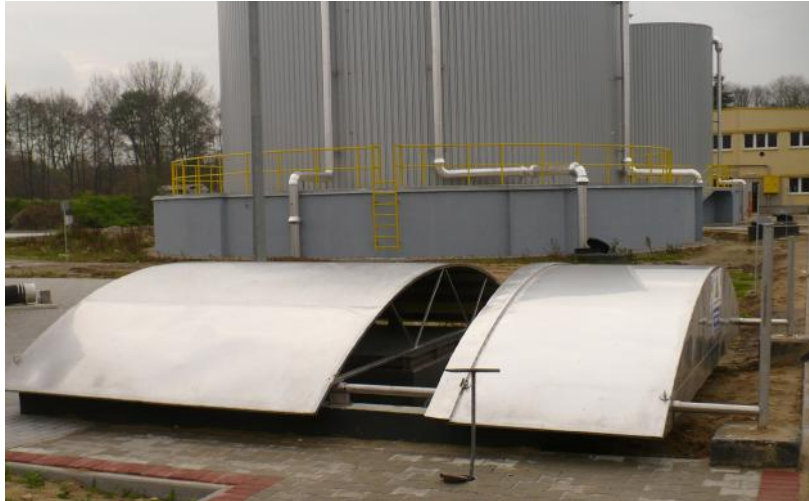
Fig. 1. View of the aboveground construction of the biogas desulphurization system using sodden ore at the Rawskie Wodociągi i Kanalizacja Sp. z o.o. company in Żydowice. Ownership of authors.
