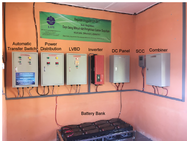
Fig. 13. The equipment of the solar electric system for Village Office and Library Building at the Seliu Island Village.
