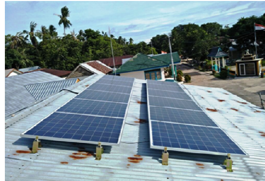
Fig. 7. PV array is mounted on the roof of the Library Building in Selu Island Village
