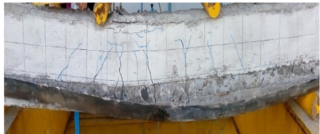
Fig. 20 Crack pattern of beam with web bonded steel plates of 4mm thick
