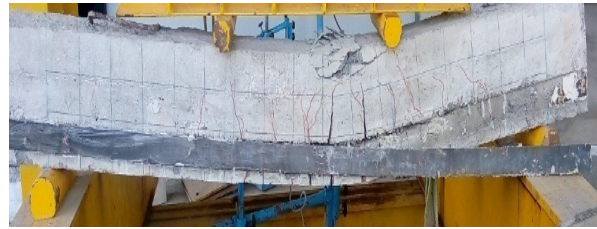
Fig. 19 Crack pattern of beam with web bonded steel plates of 3mm thick
