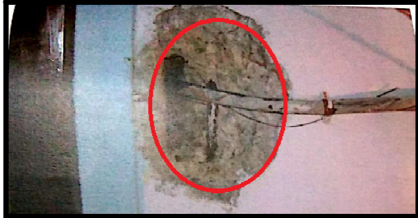
Fig.3 Showing slab breaks with exposed steel shows in red mark
