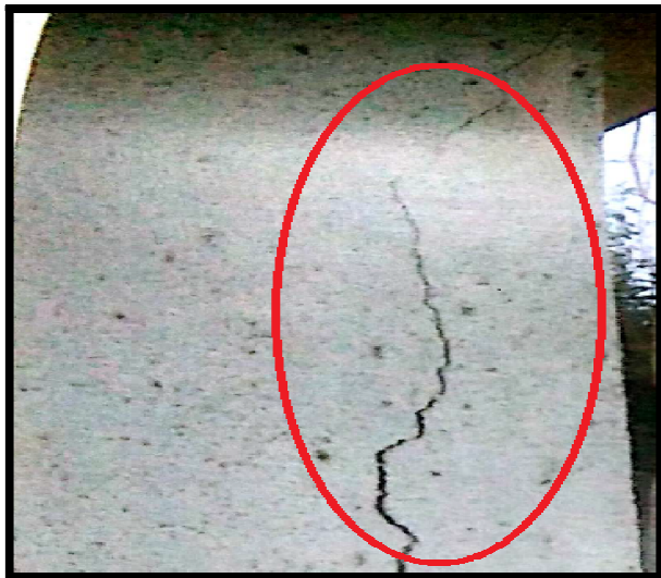
Fig. 4 Showing corner column shows corrosion cracks
