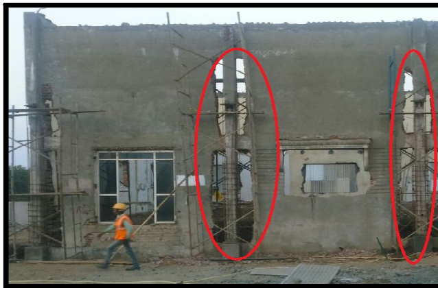
Fig. 9 Showing columns with red mark shows that they are strengthen with the help of jacketing.
