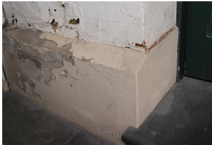
Figure 4. Rising damp exacerbated by hard cement render repairs
