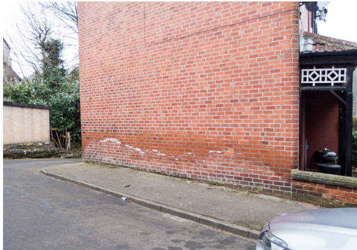
Figure 3. Rising damp on a painted brick wall
