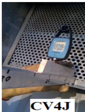
Figure 8. Discharged air jets velocity monitoring
