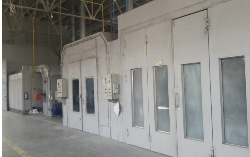
Figure 3. Dyeing / drying cabins (DDCs)
