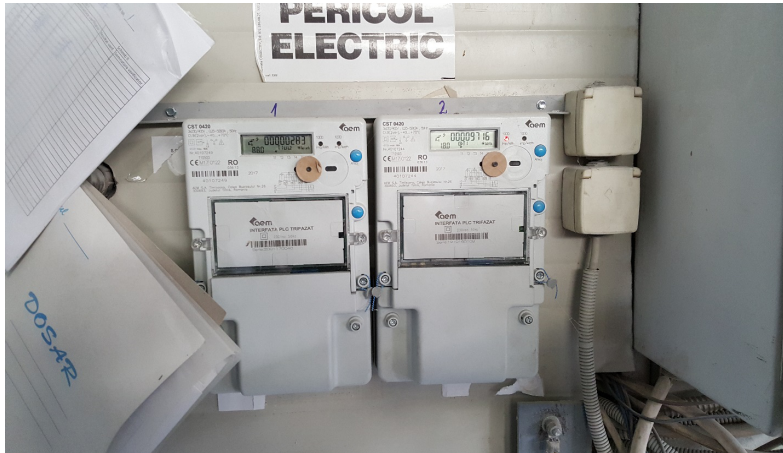
Figure 5. Electricity meters group
