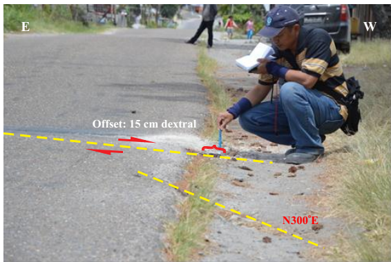
Figure 6. A photograph showing the ground surface rupture at Site 3, Jamur Ujung Village. There are two ruptures with azimuthal trends of 85° and 300°. The inferred dextral offset is 15 cm.
