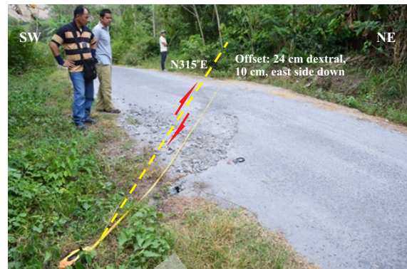
Figure 4. A photograph showing the surface rupture crossing the road between Kute Geulimai and Seurempah Villages. The rupture right-laterally displaced the road about 24 cm with a vertical displacement of about 20 cm, east side down.
