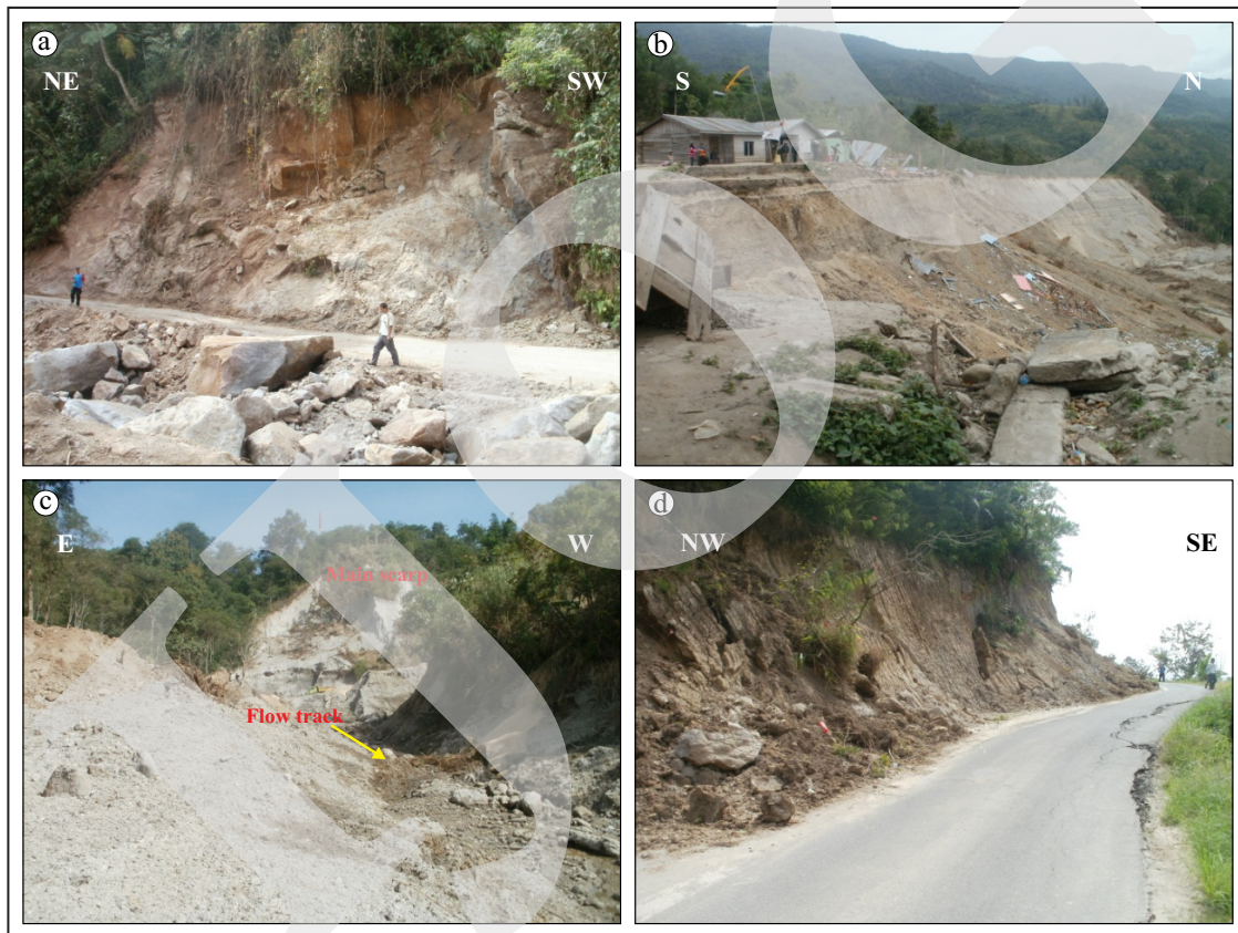
Figure 13. Photographs showing types of landslide triggered by the July 2, 2013 earthquake in a Gayo Highland area. (a) Rock fall of intrusive outcrop along the road to Kuta Panang, (b) A larger-scale landslide in Seurempah Village, (c) A dry earth flow triggered in the tuffaceous sand slope, (d) A surficial cut-slope failure along the roadside from Takengon to Blang Mancung.
