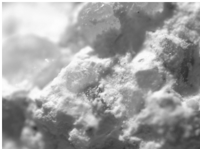
Fig. 4. The aspects of the chalk wall dried (up) and wet with efflorescence (down)
