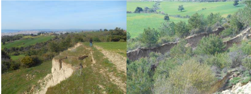
Fig. 3. Some photographs from the landslide workspace.
