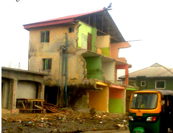
Plate 1A: severed building along Ada George road
