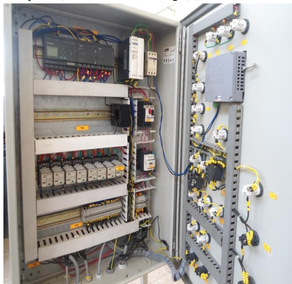
Figure 3: Electric control cabinet
