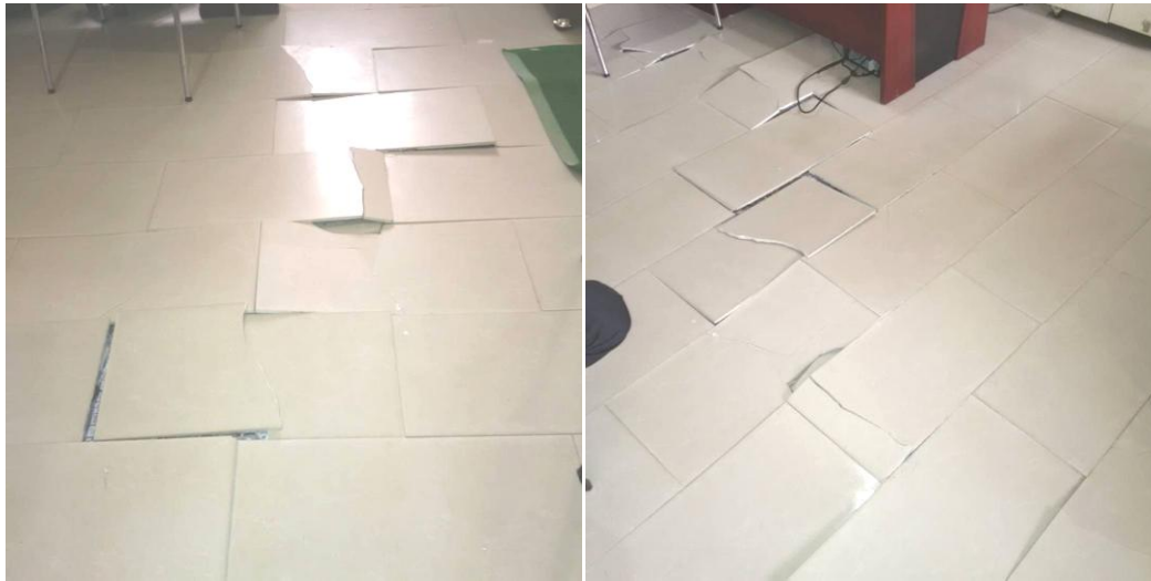
Figure 1: Structural failure of office floor, (16 th , February, 2017) showing crack lines and displacement (a) Front view (b) Back view
