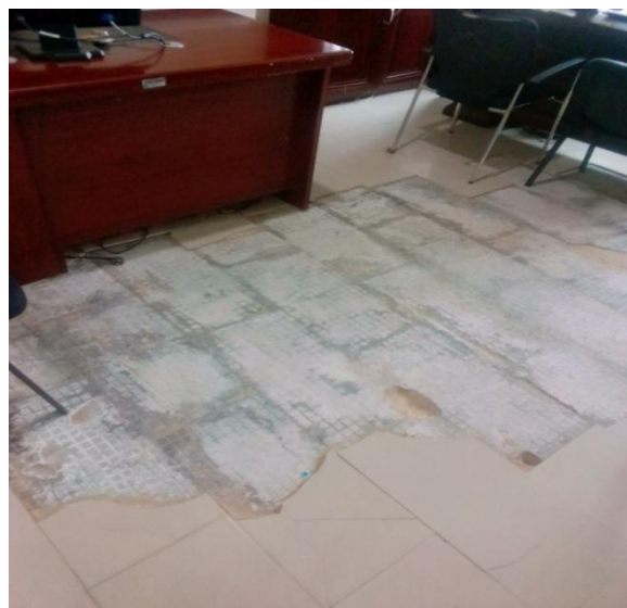
Figure 16: State of the office floor after the broken tiles were removed.
