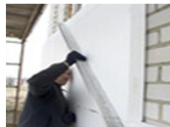
Figure 3: Wall Insulated with EPS [4]
