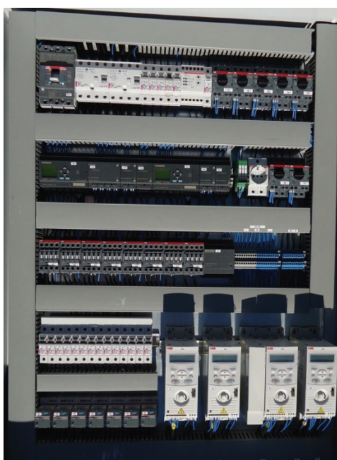
Fig. 5. The front view of the electrical cabinet for automation of the fountain.
