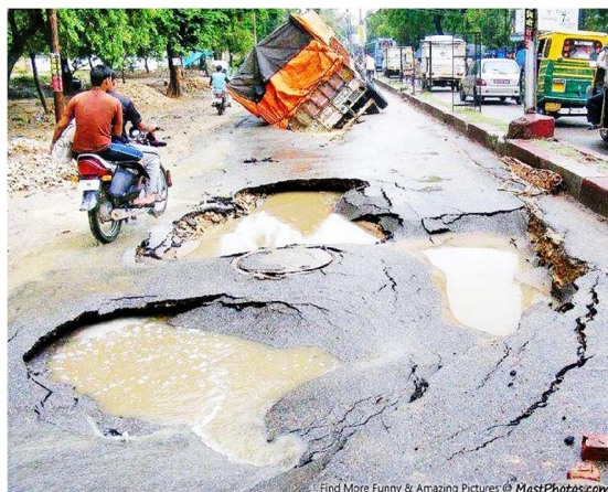
Image 5 : showing the Indian road condition in rainy season Source: http://mastphotos.com/indian-roads-rainy-season-1615.html
