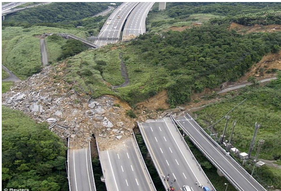
Fig. 2 Slope failure on motorway No. 3 of Taiwan (2010). For the removal of the soil, 50 excavators, 100 trucks and 1000 workers had to be used for 20 days (Source: Lee et al. 2012) [10]
