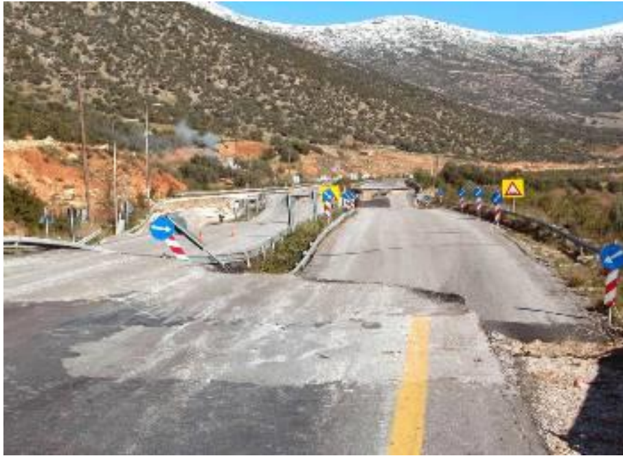
Fig. 3 The damaged road surface of the Athens-Thessaloniki National Road, from the landslide of Malakasa. (Source: https://www.google.gr/search?q=Malakasa+landslide&sa ). [13]
