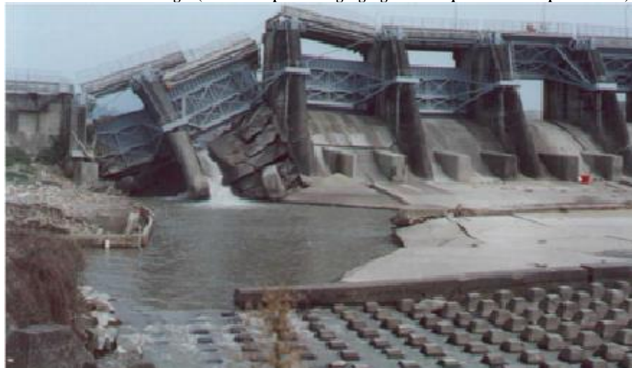
Fig. 8 Failure in the spillway of Shih-Kang Dam (Source: Wieland, 2009). [27]
