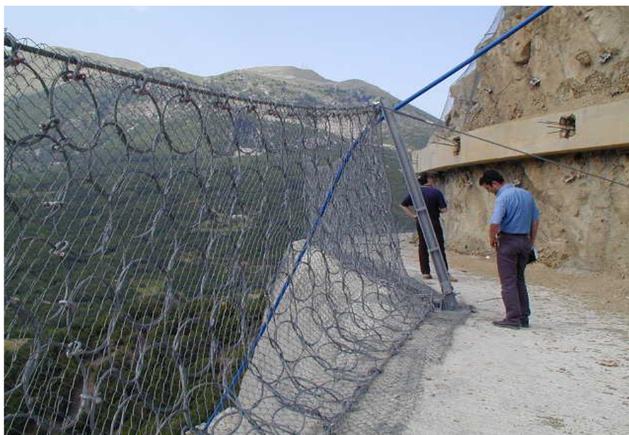
Fig. 13 Metal mesh for the protection from falling rocks. (Source: Rozos 2017). [29]
