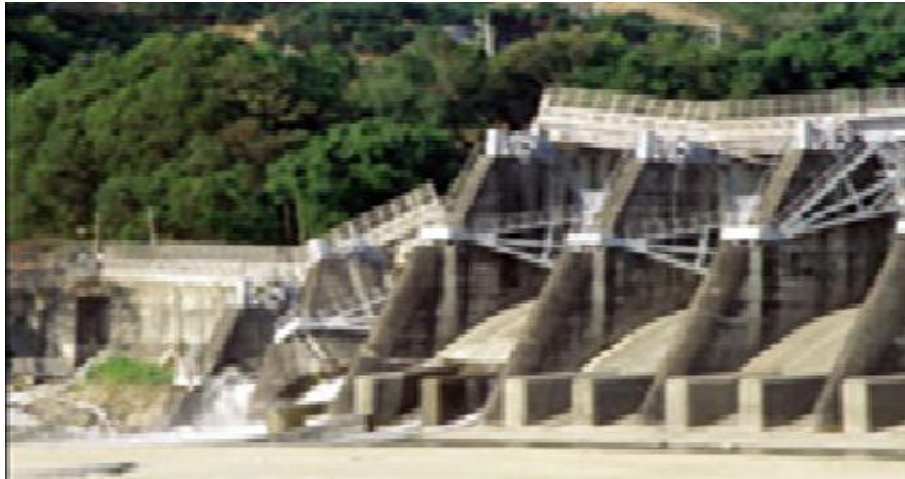
Fig. 9 Surface faulting caused major damage to the Shih-Kang Dam (Source: http://mceer.buffalo.edu/research/Reconnaissance/taiwan9-21-99/docs/lessons.asp ). [26]
