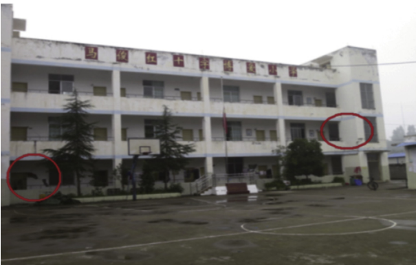
Figure 2. Majun Primary School built in 2008 after the Wenchuan earthquake and the facility was damaged on April.
