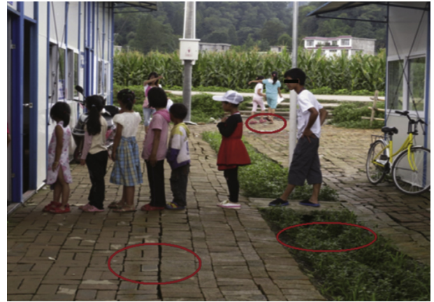
Figure 4. The uneven ground tended to result in fall-related injuries.
