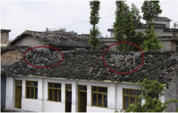
Figure 1. Gonghe Primary School built in September, 2000 and damaged on April 20, 2013.
