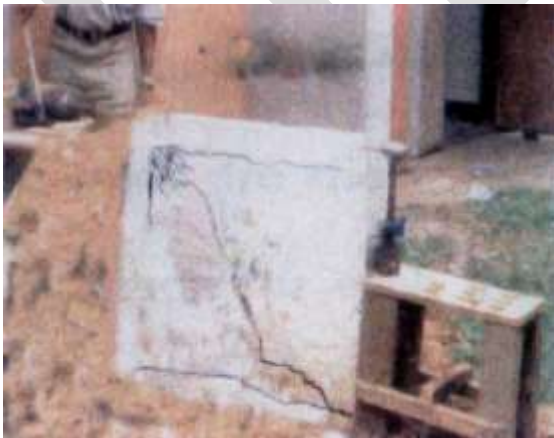
Figure 4: Failure Mode of MF2 Frame
