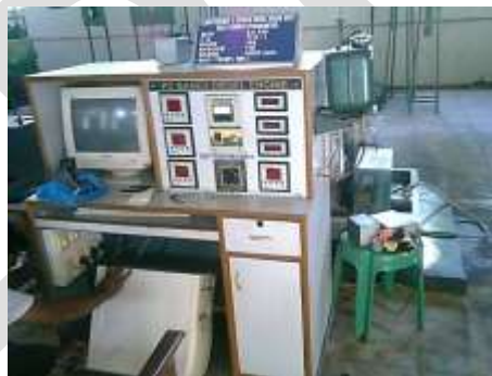
Fig 6.3: Photographic View across the Control Panel
