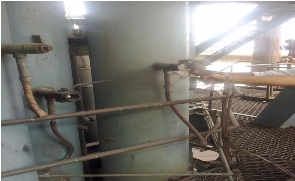
Fig 3: Velocity measurement in coal pipe.
