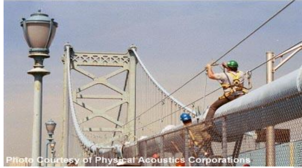
Figure 2 inspection for in-service damage
