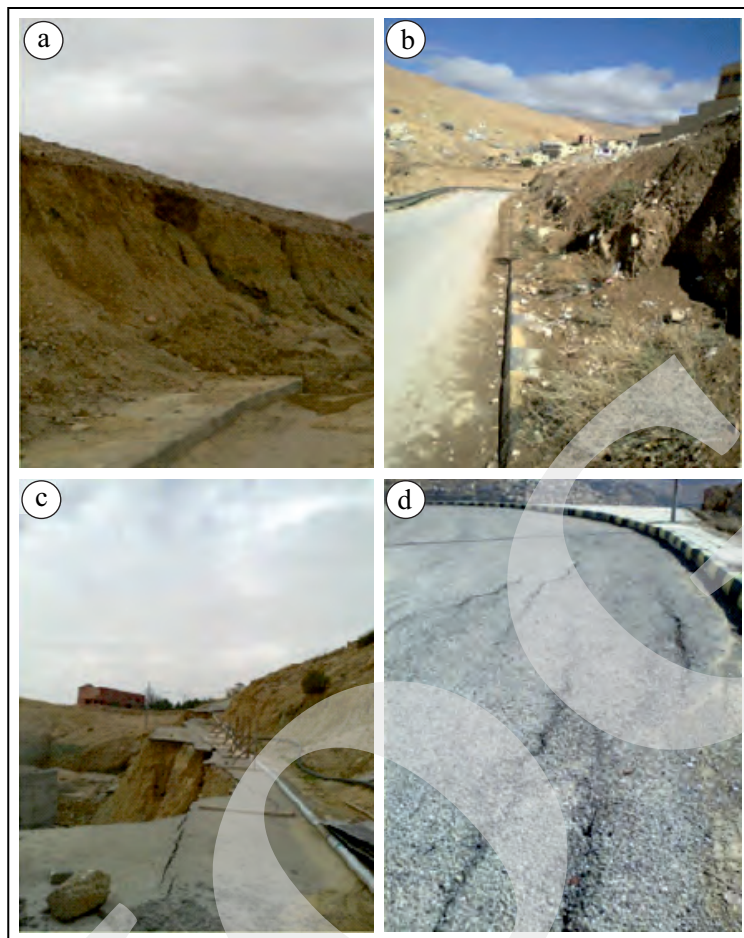
Figure 5. Registered landslides (a, c) and erosions (b, d) in the streets and roads of the studied area.
