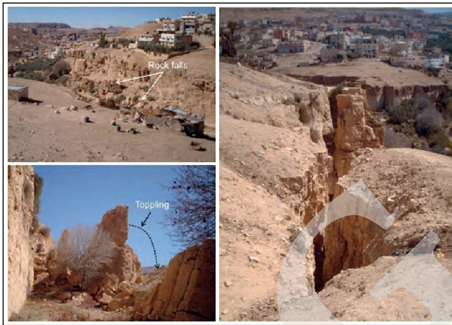
Figure 4. Toppling and rock falls in the studied area.
