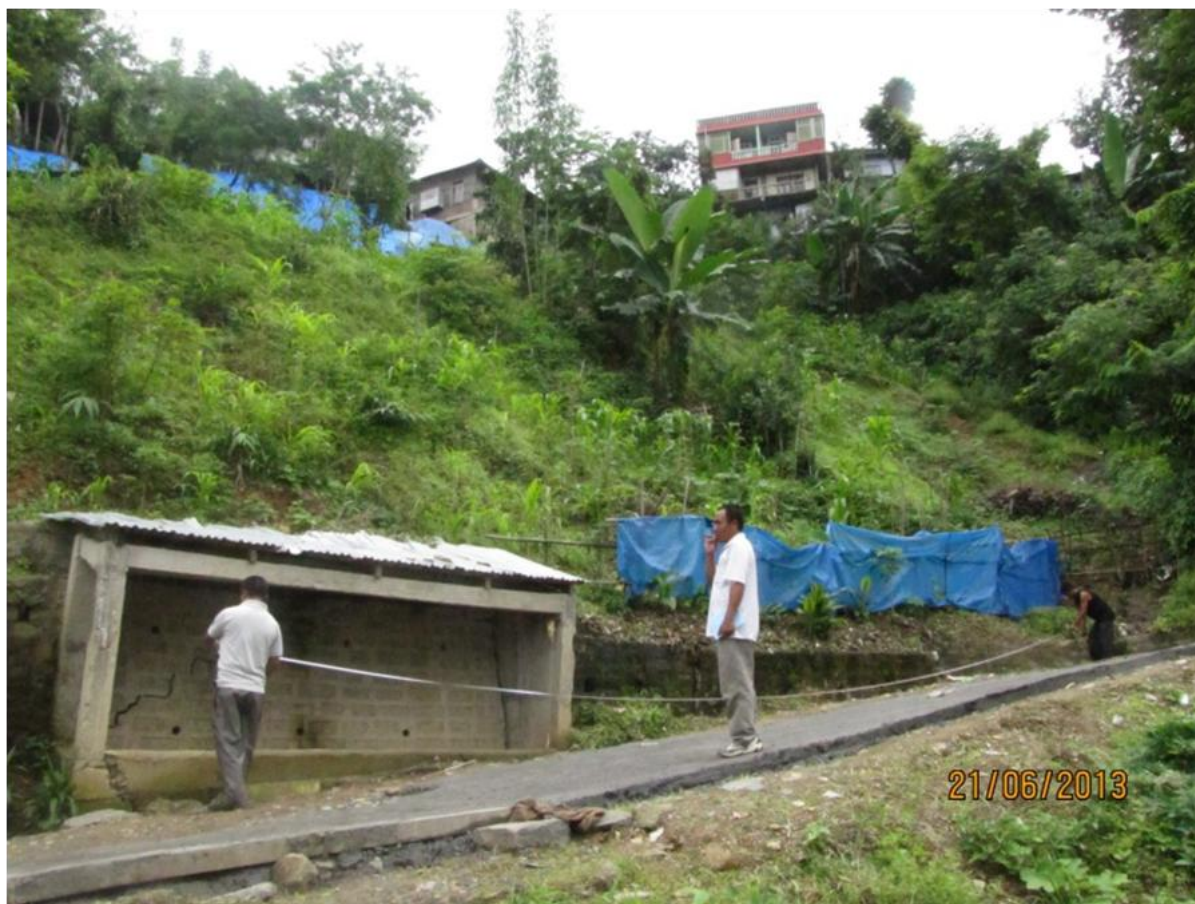
Photo plate 5. Proposed reconstruction of Cheinal chava drain, and breast wall at New Colony- I & III locality.
