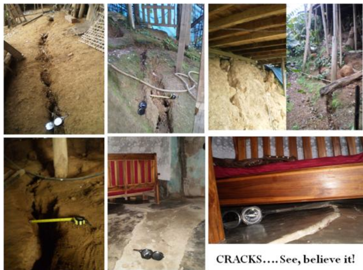
Photo plate 2. Some of the cracks observed at the settlement of New Colony & College Veng slumping areas.
