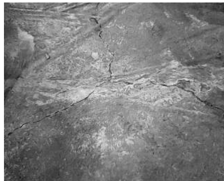
Plate 1: Typical Plastic Shrinkage Crack
