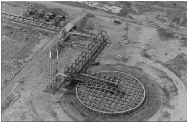
Figure 2: Photo of the underground LNG tank (GL4/Z complex, Arzew – Algeria)
