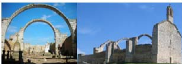
FIG. 5 THESE IMAGES SHOW THE STATE OF THE CHAPEL THAT NEEDS AN INTERVENTION FROM WHICH A DIALOGUE IS IMPLEMENTED FOR LEARNING
