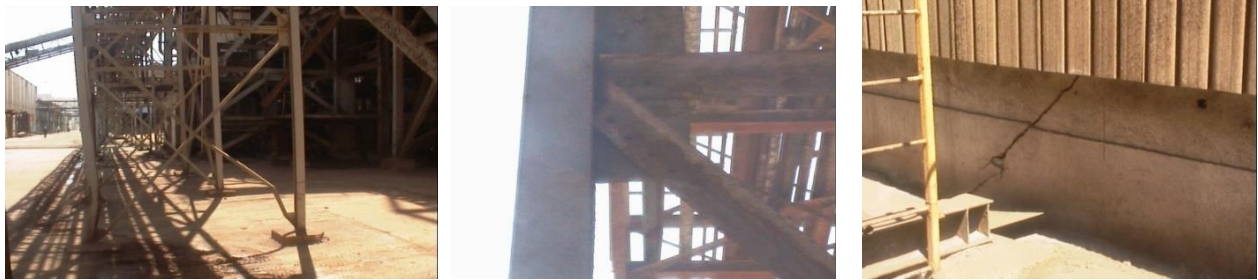
Fig. 6 –Deformation of the bracing system, lack of bolts in the joints and 45 degree cracks in both directions of the joint
