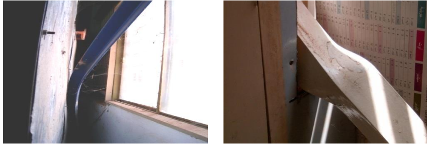
Fig. 9 –Instability phenomenon on the bars of the bracing system
