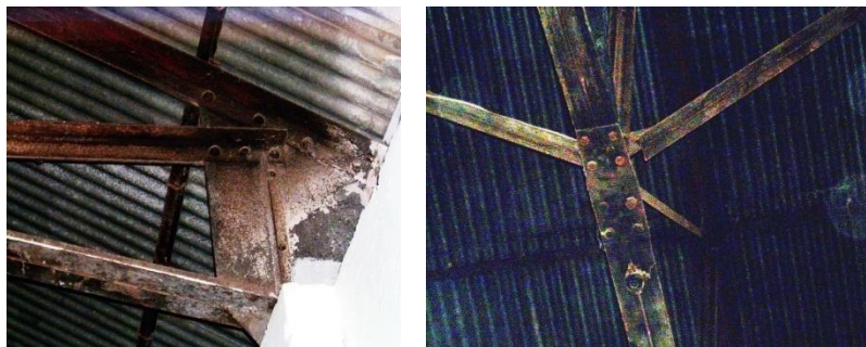
Fig. 11 –Advanced corrosion of bearing parts and assemblies
