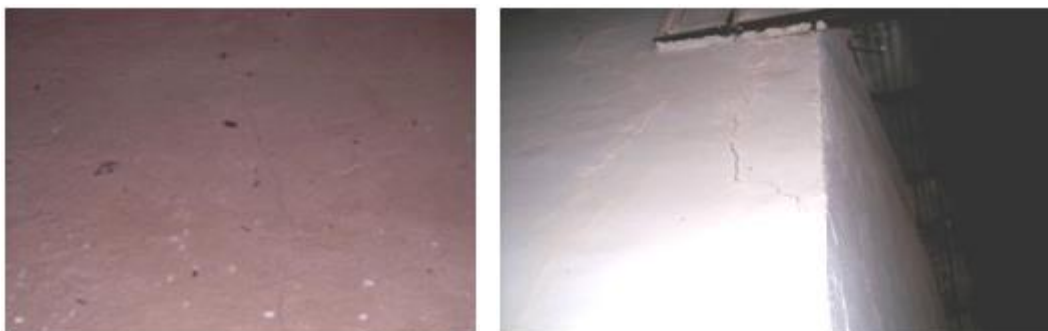
Fig. 12 –cracks in walls and pavements
