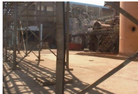
Fig. 7 –Buckling of columns
