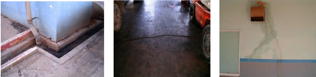
Fig. 10 –Soil subsidence, cracks at the base of walls in pavements and walls
