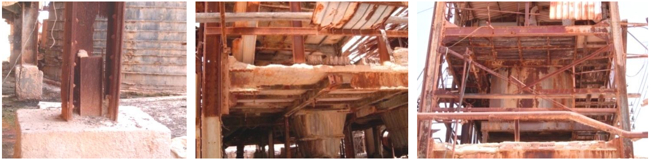
Fig. 5 –Degradation of the bracing system and advanced corrosion
