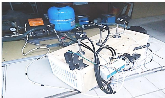
Figure 2. Photo of the exterior of the heat exchanger housing and the complex, including a circulation pump, a hydraulic accumulator, a balancing valve and an electromagnetic fluid flow converter.
