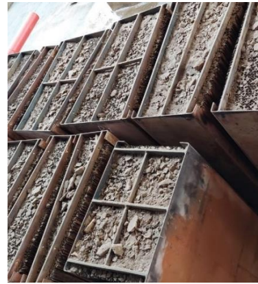
Figure. 13 Finding of plugging in air preheater element during overhaul inspection
