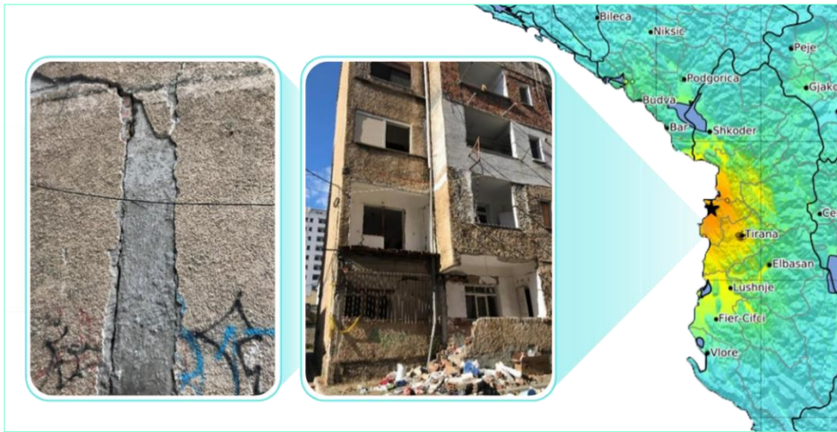
Fig. 3 Location of the damaged template design building considered in this study with respect to epicenter of November 26, 2019 earthquake.
