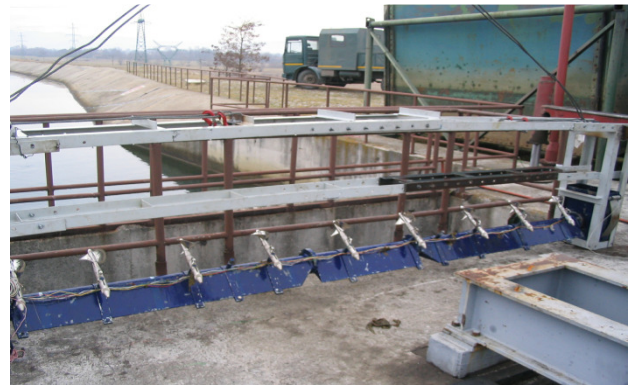
Fig. 3. Hydraulic frame used to place the current meter
