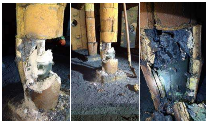
Figure 3. Damages occurred at the vertical girders
