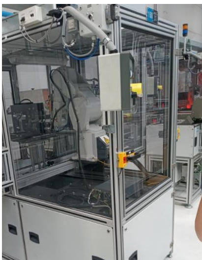
Fig. 1. Fencing of a robotic workplace
