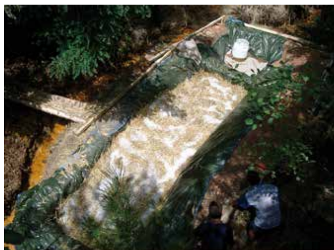
Fig. 10. Treatment of acid mine drainage by means of permeable reactive multibarrier in the Kurilo deposit
